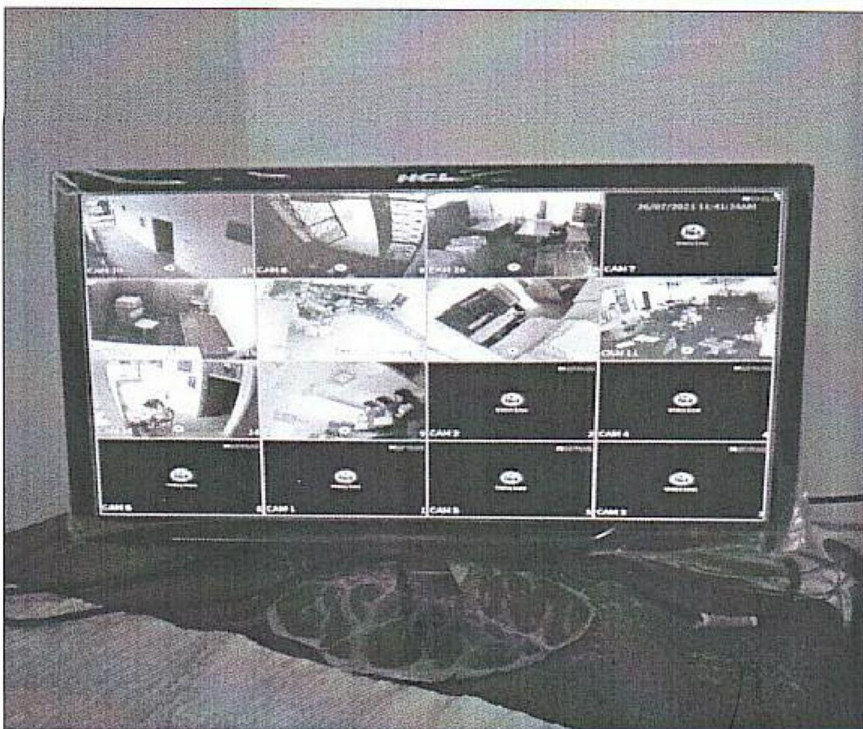
Photograph of CCTV
